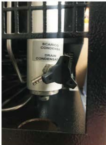
The two drain taps to keep condensation out.
